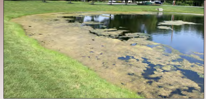
A stormwater pond being evaluated for excessive algal growth
