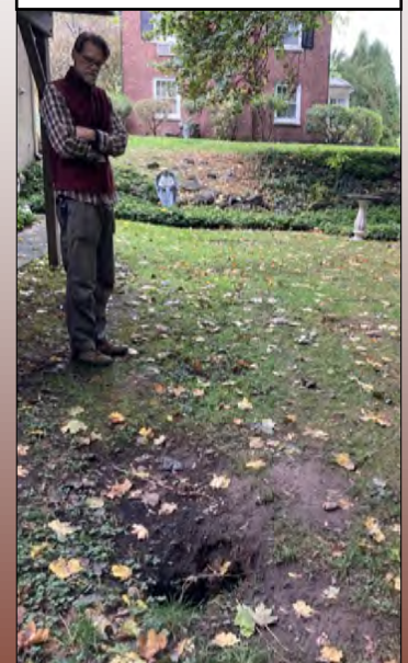
Sinkhole from stormwater runoff
