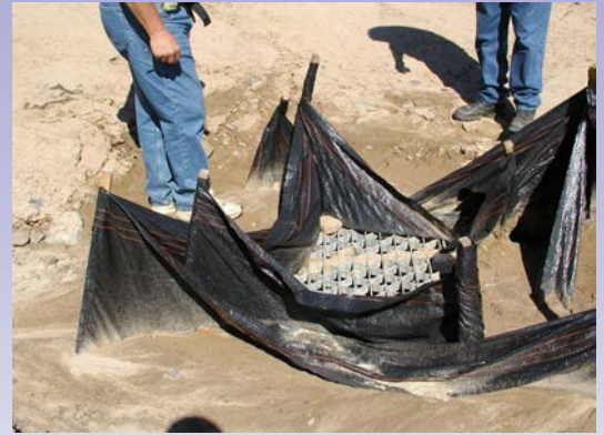
A poorly installed inlet protection;, anything flowing on the construction site will be washed into our rivers and streams
